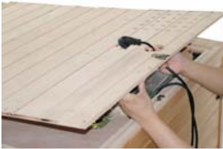
FIG-23 Slip the power plug through external top board
